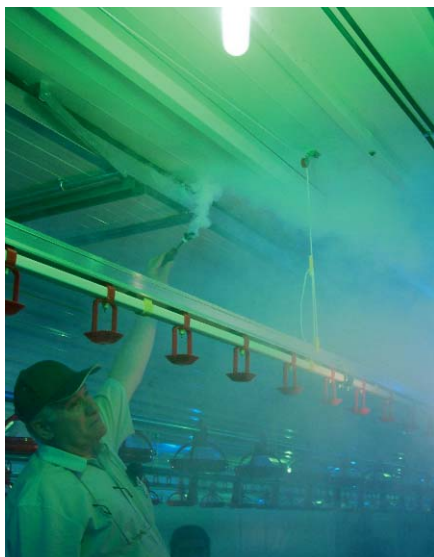
Smoke trials showed that air is distributed quickly and efficiently over the whole house.
