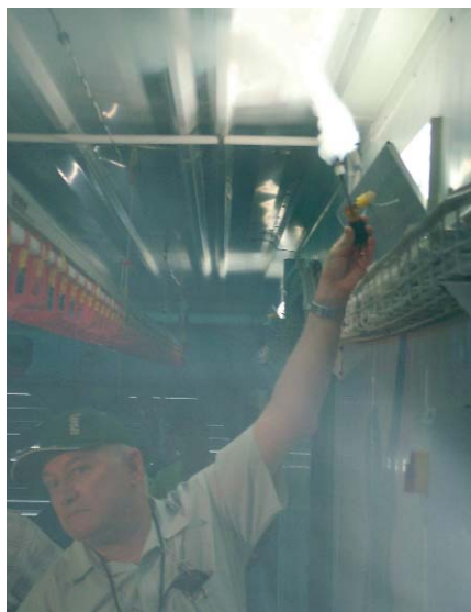
Controlled side wall inlets allow good air distribution during minimum ventilation.
