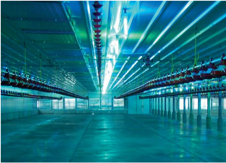
Wide houses require air inlets in the ceiling to refresh the air in the middle of the house.
