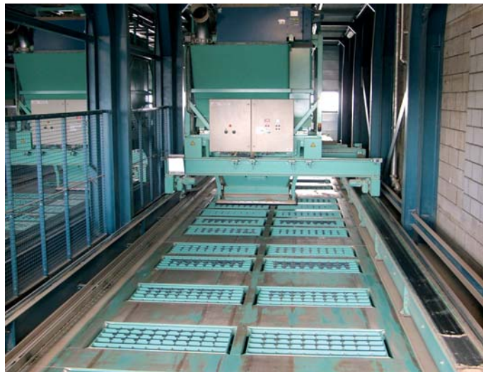
The contrasets are filled by a moveable weighing systems that can move forward, backward and sideways to reach every opening.
