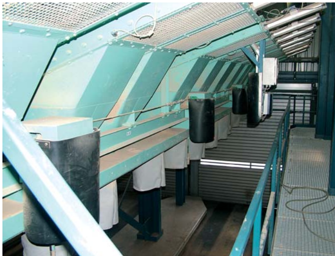
Top view of the contrasets for immediate loading of a bulk truck.
