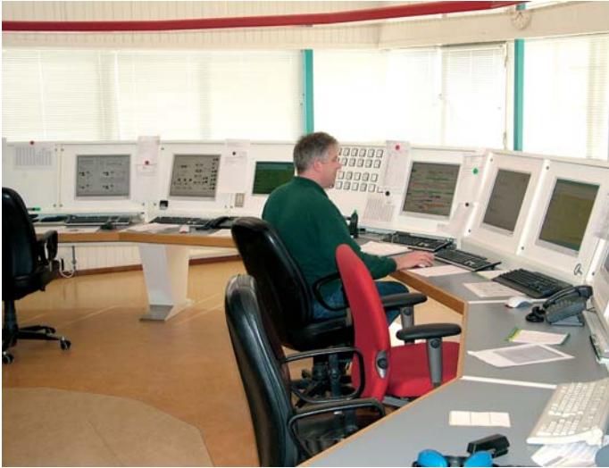
Production, supply and delivery is controlled from this room, where two people manage the whole mill.
