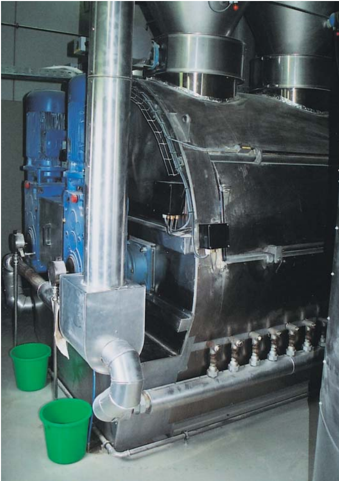
Forberg heated mixer for sanitising the feed.
