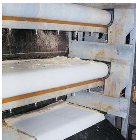
As soon the broilers are ready for processing, belts transfer them to the end of the structure where they are separated from the litter. The birds and litter are transferred respectively to the loading platform and litter containers/storage.
